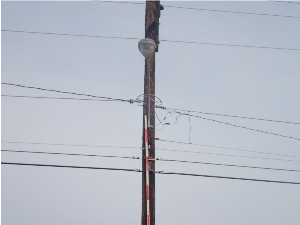
Figure 3 - Ungrounded Luminaire clearance to communication cables
